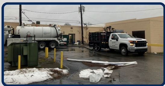
Leaking Transformer Behind Business
